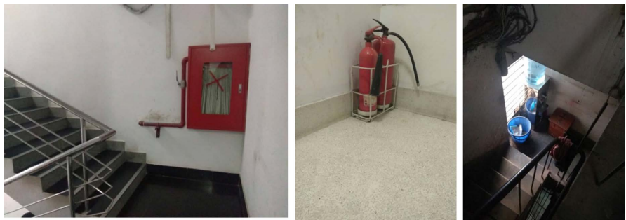
Figure 12. Firefighting appliances & additional escape route at HBR tower.
