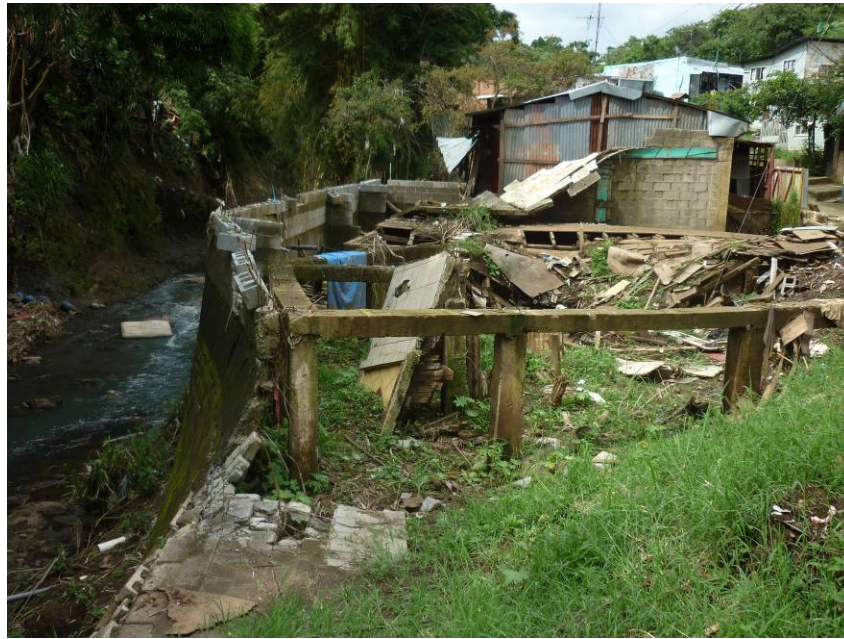
Figure 3. Damage in Barrio Fátima caused by the flood of 2010. Courtesy of Oscar Sojo
