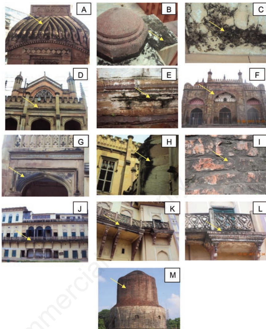
Figure 2. Historical monuments of Varanasi, India, showing surface colonization of cyanobacteria. (A) Brahaspati Temple, (B) Vishwanath Temple, BHU, (C) Bharatmata Temple, (D, E) Madhavrav's Dharhara, (F-H) Sanskrit University, (I) Jalnigam's old tank, (J-L) Ramnagar Fort and (M) Dhamek Stupa, Sarnath.
