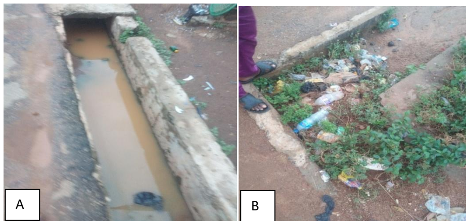
Fig. 9A. Water logged drainage at Araromi, B: Blocked Drainage at Owode Source: Author's Field Survey, 2022
