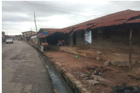
Fig. 8. Dilapidated Corrugated Iron Sheet for Building Construction at Araromi Source: Author's Field Survey, 2022
