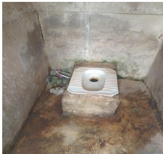
Fig. 6. Pit Latrine with Modern Squat-Bowl at Oja-Oshodi Source: Author's Field Survey, 2022
