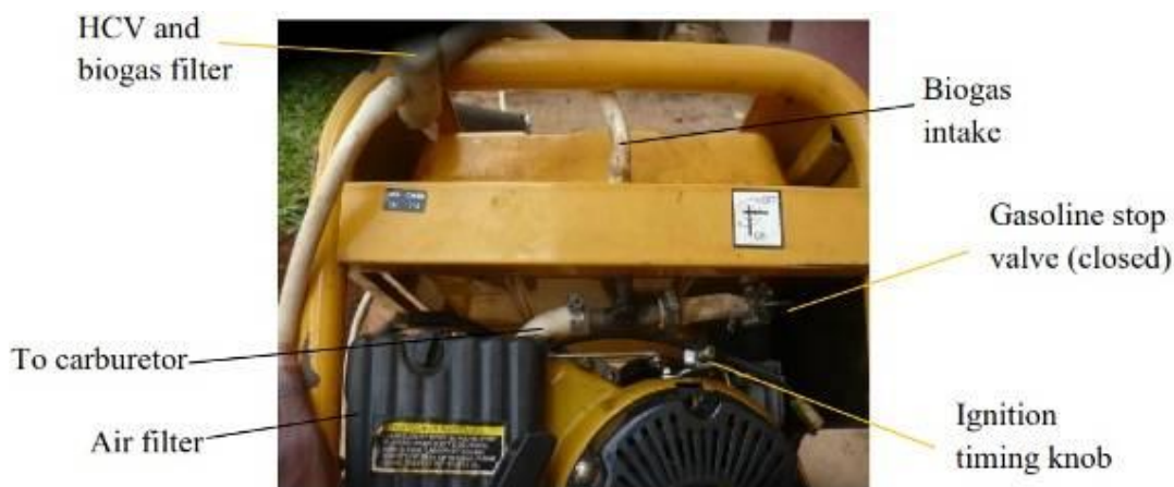
Fig. 4. Metering set mounted on the electricity generator set
